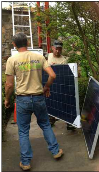
Installation of solar panels begins! Photo courtesy of UU Church of Chattanooga
